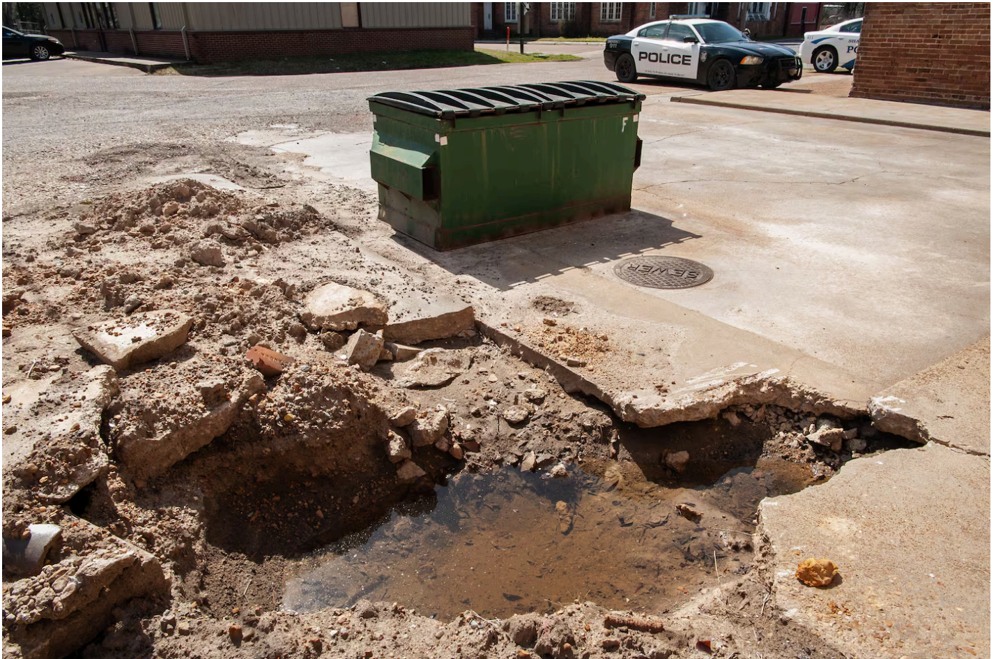
Unfinished pipe repairs remain near city hall. RORY DOYLE FOR THE BOSTON GLOBE
